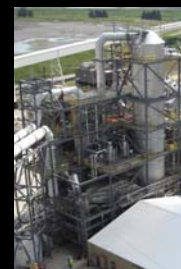
20 MW capture unit at AEP's Mountaineer Power Plant (West Virginia)
