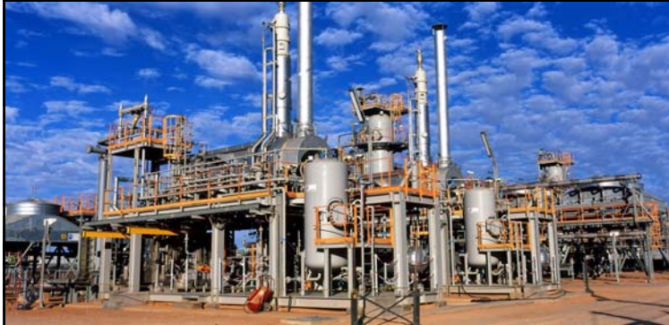
BP Natural Gas Processing Plant (In Salah, Algeria)
